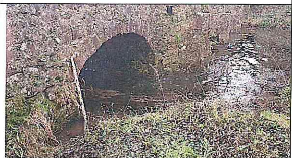
Photo 6 Flood damaged masonry on Mill bridge (3/1/2020)
